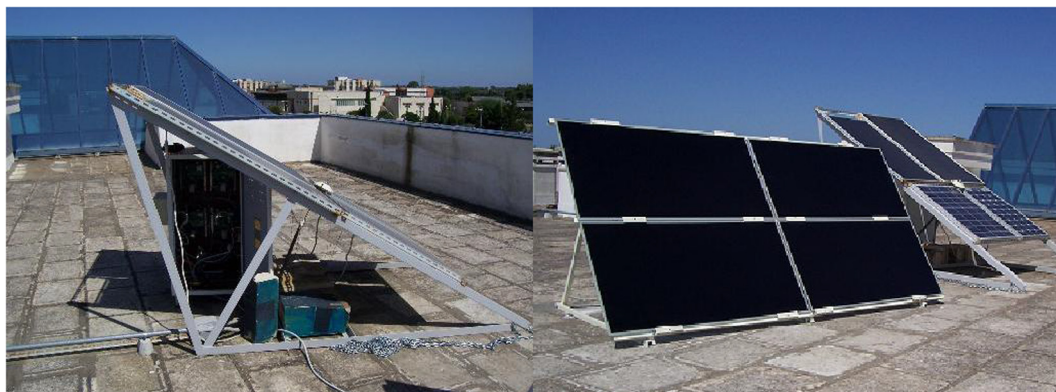
Fig. 3. View of thin-film CdTe PV modules located on the Dept lab roof.
