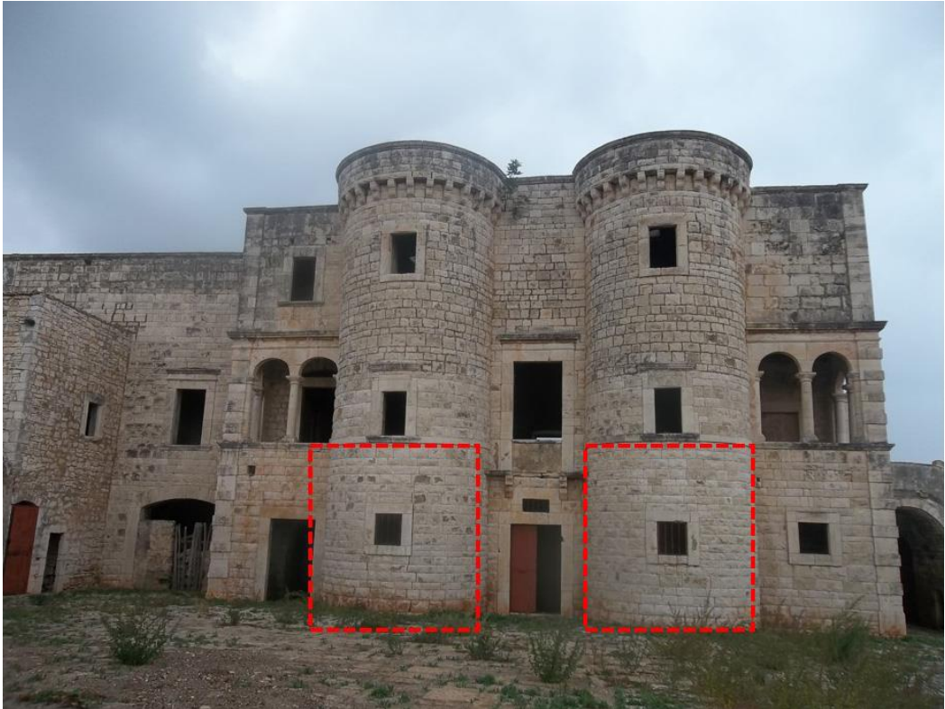
Figure 4.7-1 Picture of crack patterns of the southern wall.
