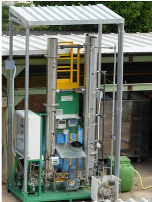
Fig. 2.5.1. A photograph of the SBBGR treatment plant.
