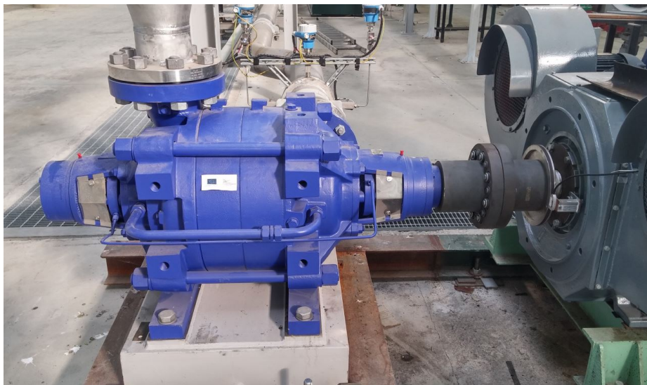
FIGURE 3.12: The booster pump of the Test Rig.
