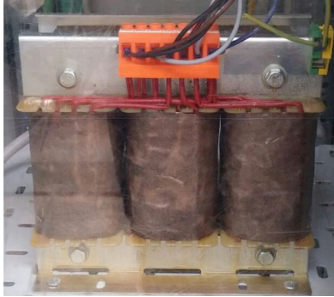
FIGURE 3.7: 380/230 VAC - 3 phase transformer.
