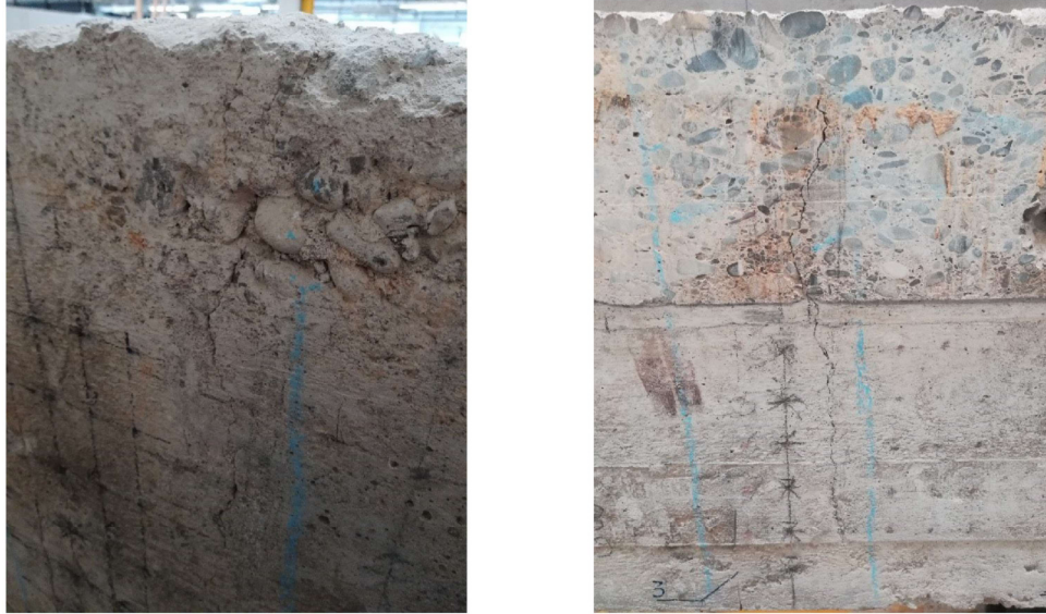
FIGURE 3.84: Crack detail: on left side, crack F3; on right side, crack F4
