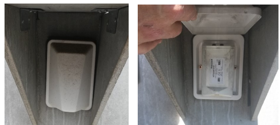
Figure 5: Honeywell - H7508A1042 - Outside Air Humidity Sensor. Apolonio Morales 29, Madrid, Control System. Source: Self-elaboration.
