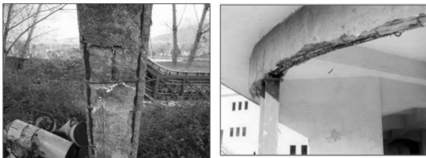
Fig. 7.4 – Examples of highly corroded existing columns, so that reinforcement bars are exposed (from Iovino et al. (2014))
