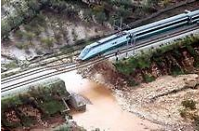
Figure 2.16 Railway embankment after 2005 flooding event, Acquaviva Delle Fonti city (BA)
