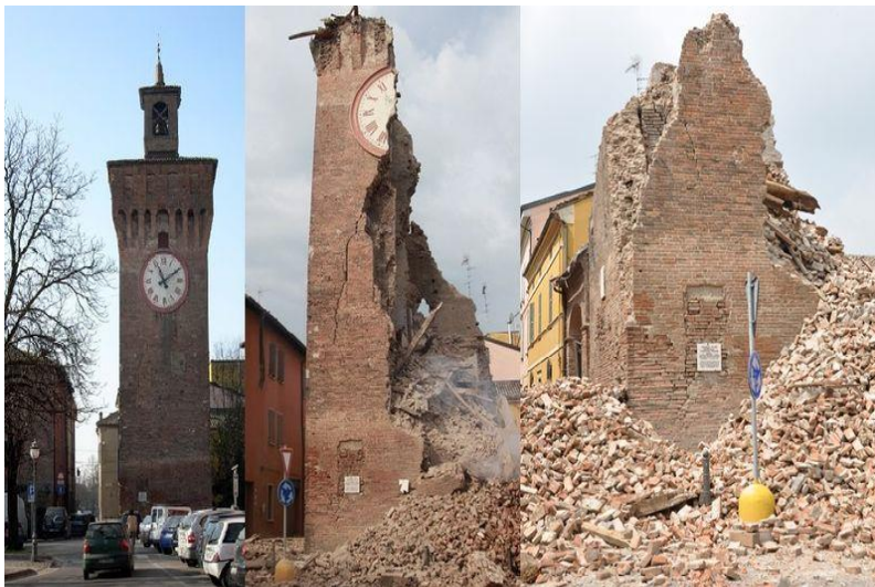
Fig. 1. 3 – Collapse of the Finale Email Clock Tower (Italy) after the May 2012 Emilia Romagna earthquake sequence.
