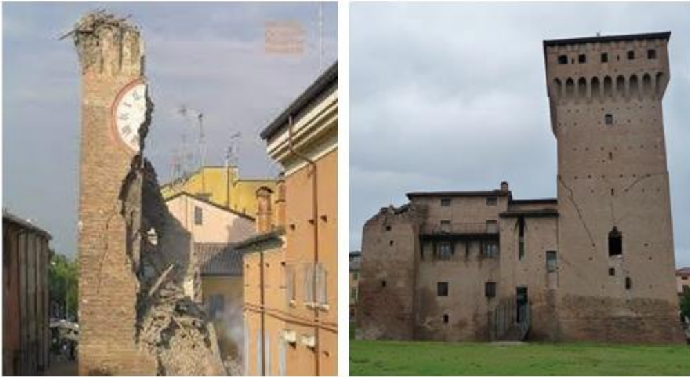
Fig. 2. 11 – a) Vertical splitting collapse for the “Clock Tower” located in Finale Emilia; b) “Heyman type” mechanism for the “San Felice sul Panaro Tower” located near Modena.
