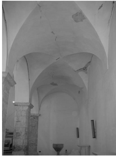
Figure 2-1. Church of San Giuliano di Puglia in Campobasso (Italy). Seismic damage (2002 Earthquake) at global scale of masonry cross vaults.
