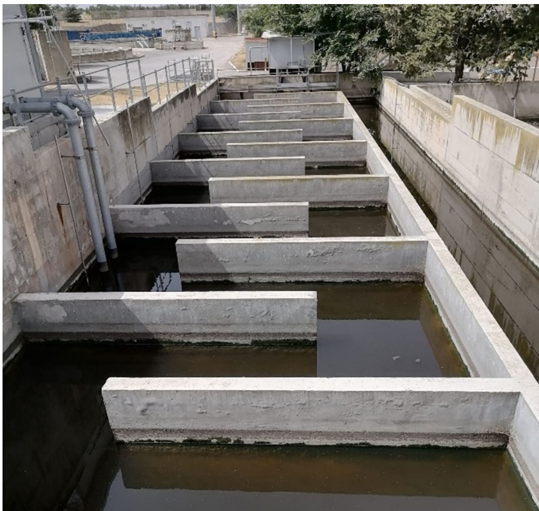
Figure S8. Disinfection tank.
