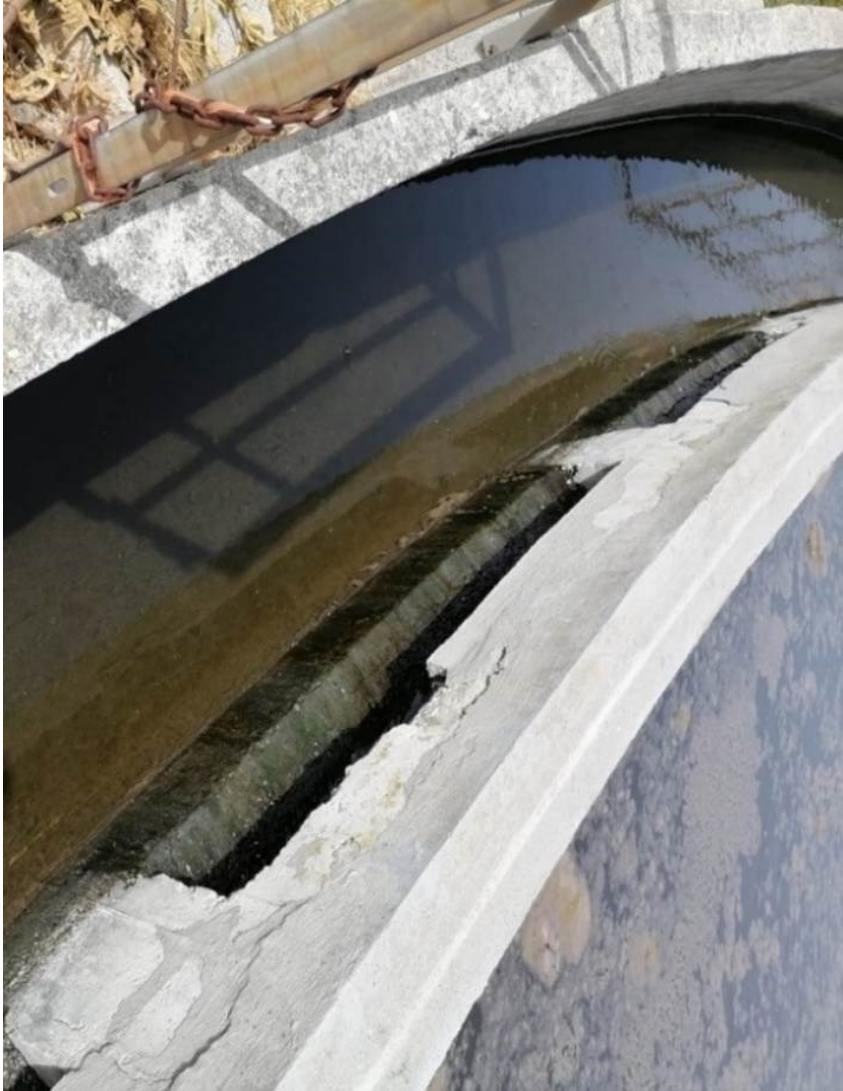
Figure S4. Weir outlet section of a sedimentation tank.
