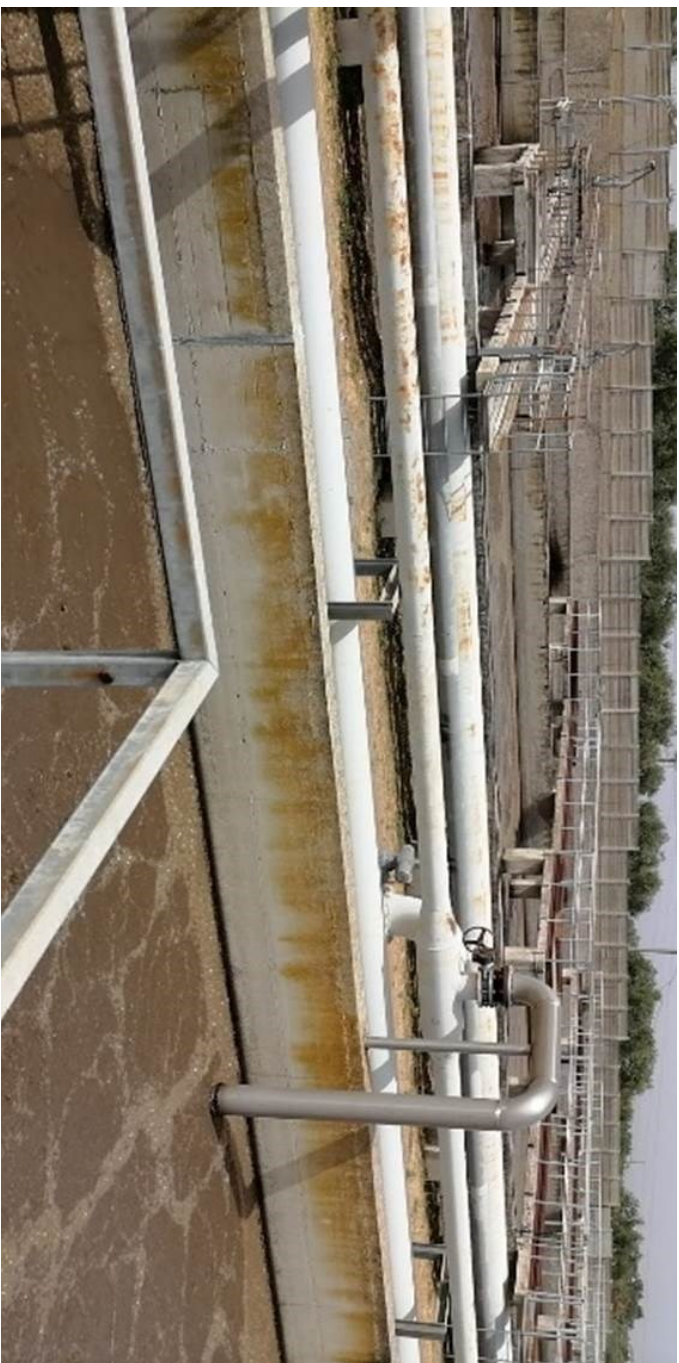
Figure S6. Aeration system of activated sludge treatment.
