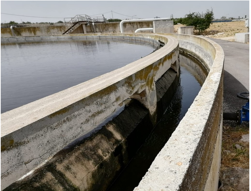
Figure S7. Wastewater after secondary sedimentation.
