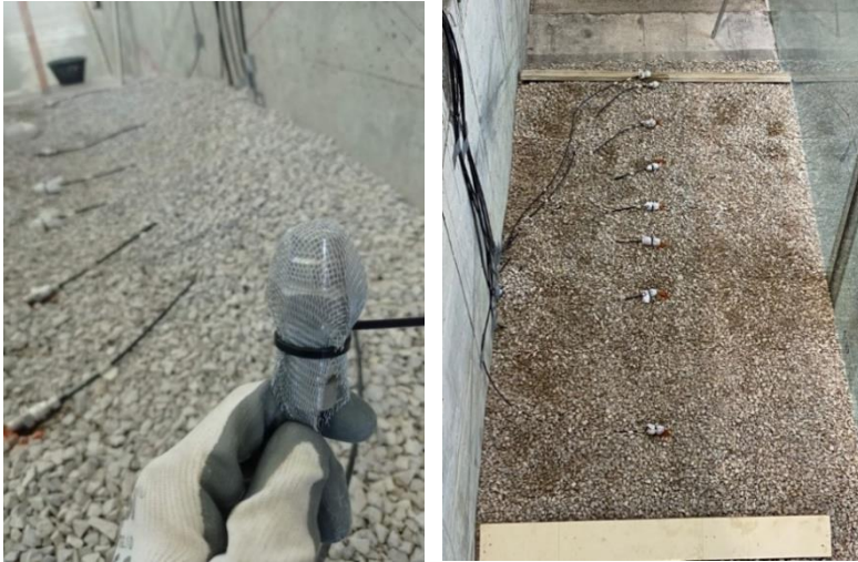
Figure 18: Installation phase inside the core of the rubble mound breakwater of pore pressure sensors.
