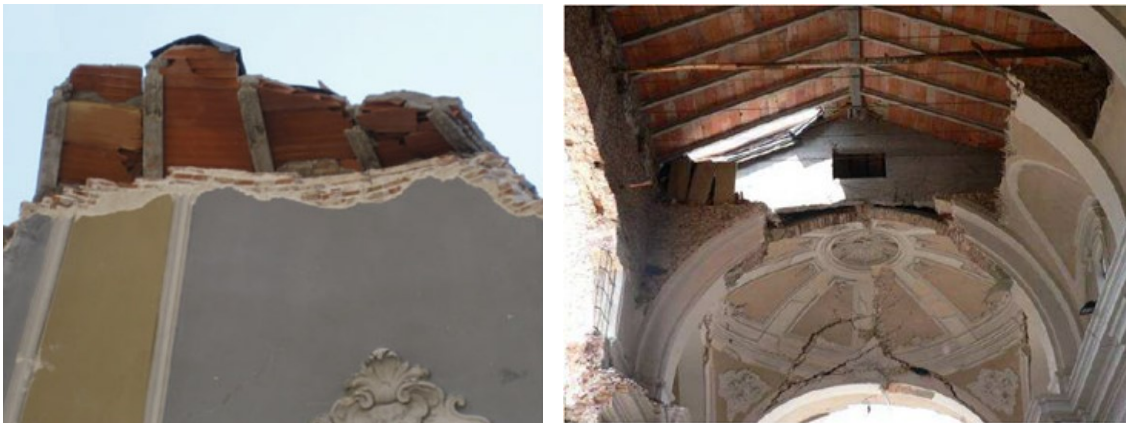
Figure 14: The modern roof made by precast elements and unreinforced concrete slab in Santa Maria Paganica church in L'Aquila [5], inside view of San Marco church in the historical centre of L'Aquila [4]
