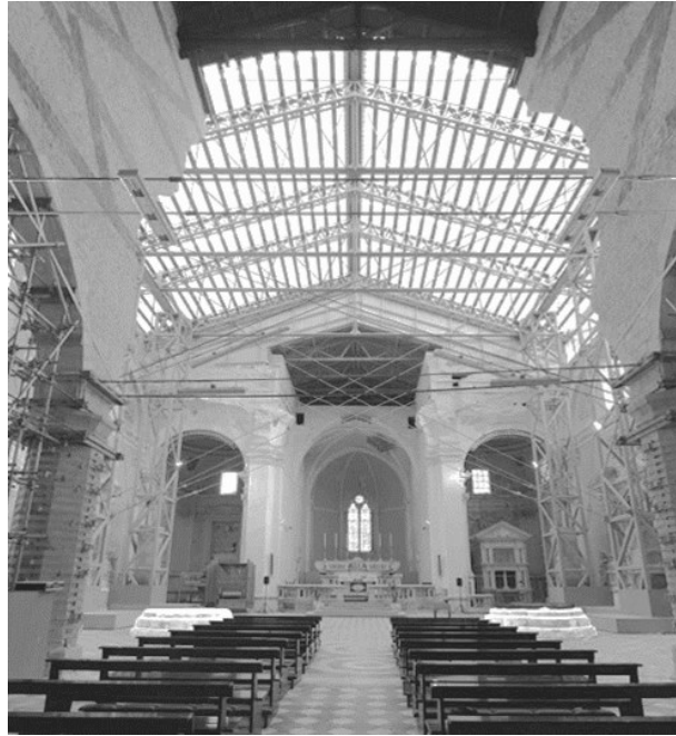
Figure 16: The basilica of Santa Maria in Collemaggio after the L'Aquila earthquake in 2009.
