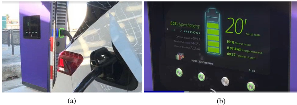
Figure 2.39: HPC fast charging station ready to operate (a) and operation panel of the station (b).
