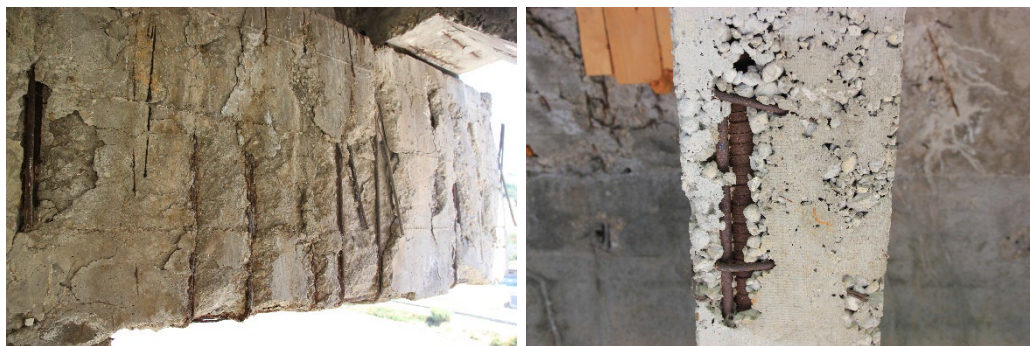
Figure 7 - Degradation of concrete structures.
