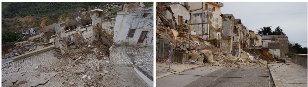
Fig. 64 - Observed damages on buildings and roads.
