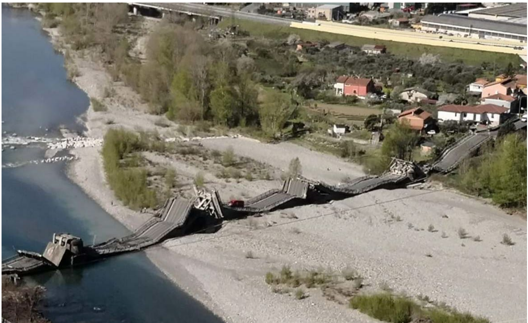
Fig. 2 - Collapse of a bridge in Albiano Magra (Massa-Carrara, Italy), 8th April 2020, (Delle Luche, 2022).
