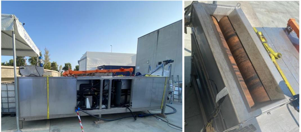
Figure 20 – DRYWA dryer and detail of the loading hopper
