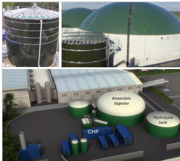
Figure 19 – Hydrolysis tank and anaerobic digester in the AD area of TERSAN plant
