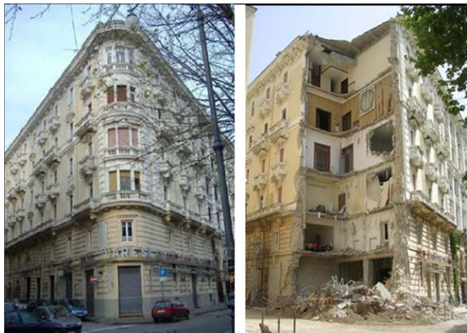
FIG. 1—The building corner before and after the collapse.
