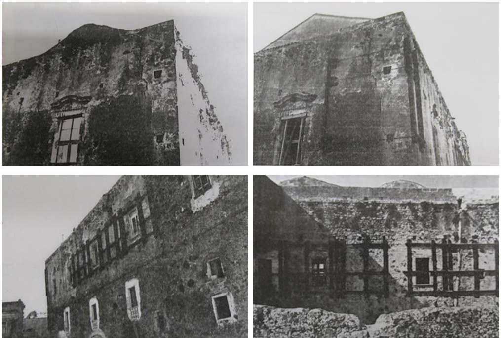
Fig. 75 Photos of the report of the project of the 29.06.1991:Consolidation works realized in in the period 1980-1985
