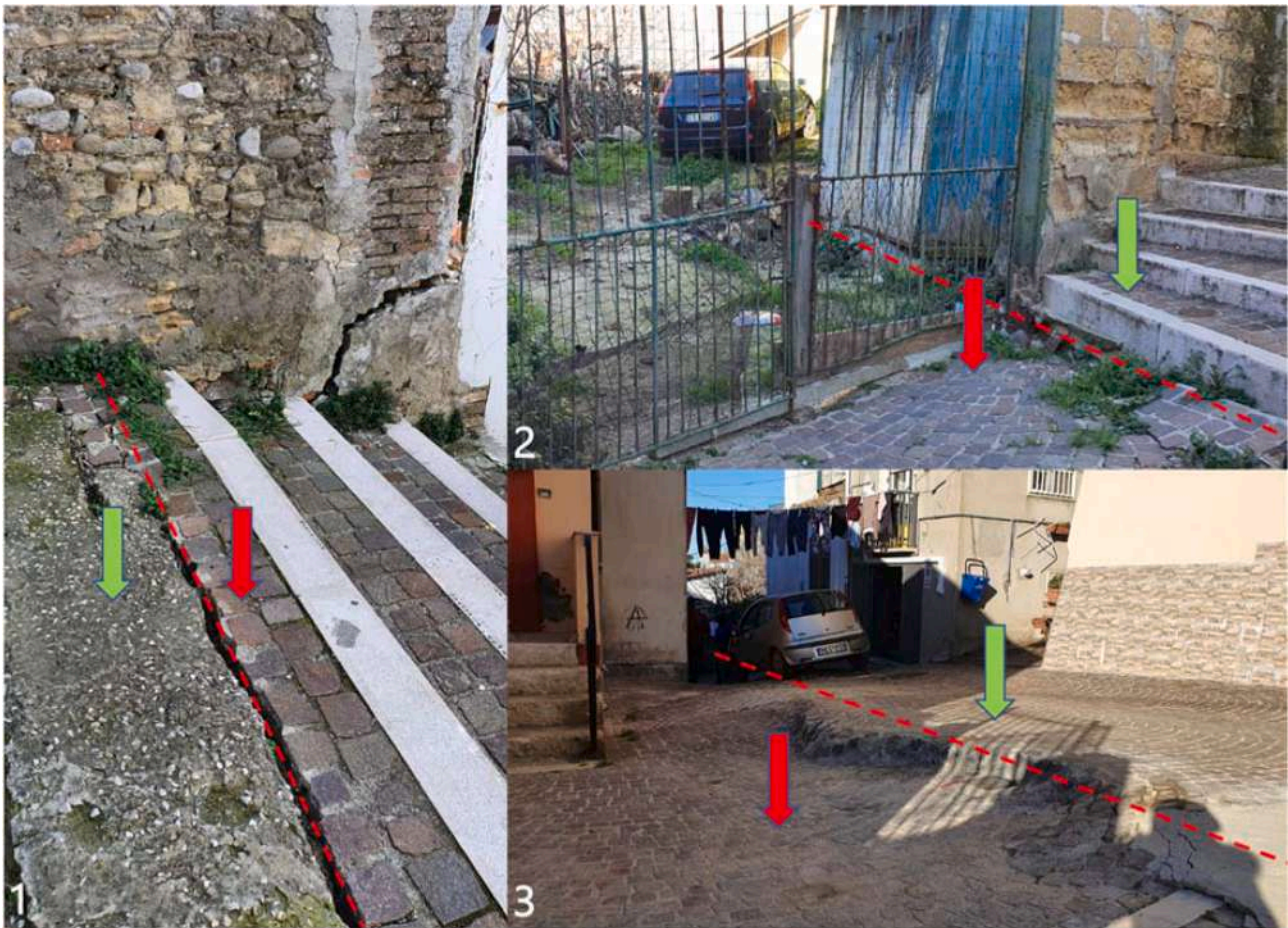
Fig. 7. Damages caused by differential displacements between the stable (indicated with green arrows) and unstable area (highlighted with red arrows) on 1) Via Bianchi, 2) via De Figlia and 3) Via Tumolo. (For interpretation of the references to colour in this figure legend, the reader is referred to the web version of this article.)
