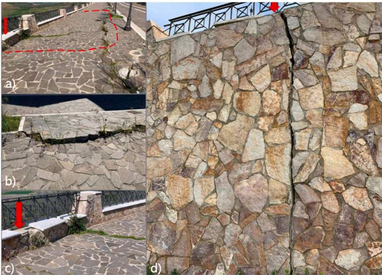
Fig. 6. Damages on the retaining wall (indicated by the red arrow) and the adjacent sidewalk. The dashed line borders a) the sector location of a marked subsidence compared to the surrounding area, displayed in b) and c). (For interpretation of the references to colour in this figure legend, the reader is referred to the web version of this article.)
