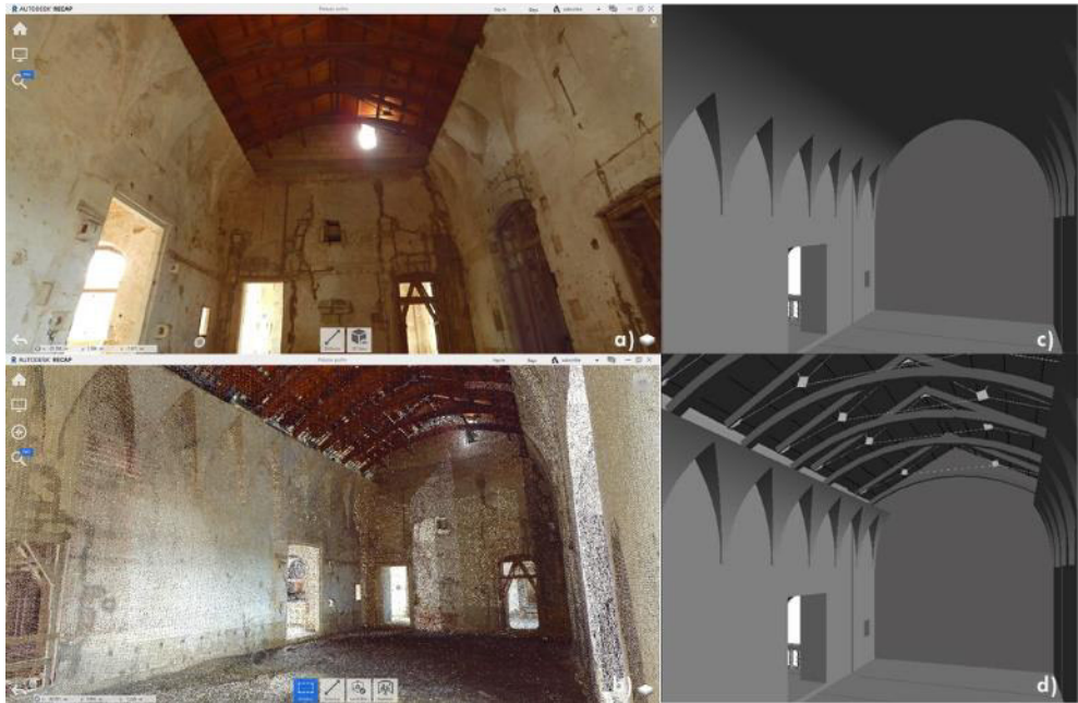
Fig. 93 Internal environment of the building which suffered the collapse of the vault a) and b) point cloud views, c) the old vault, d) the current roof.
