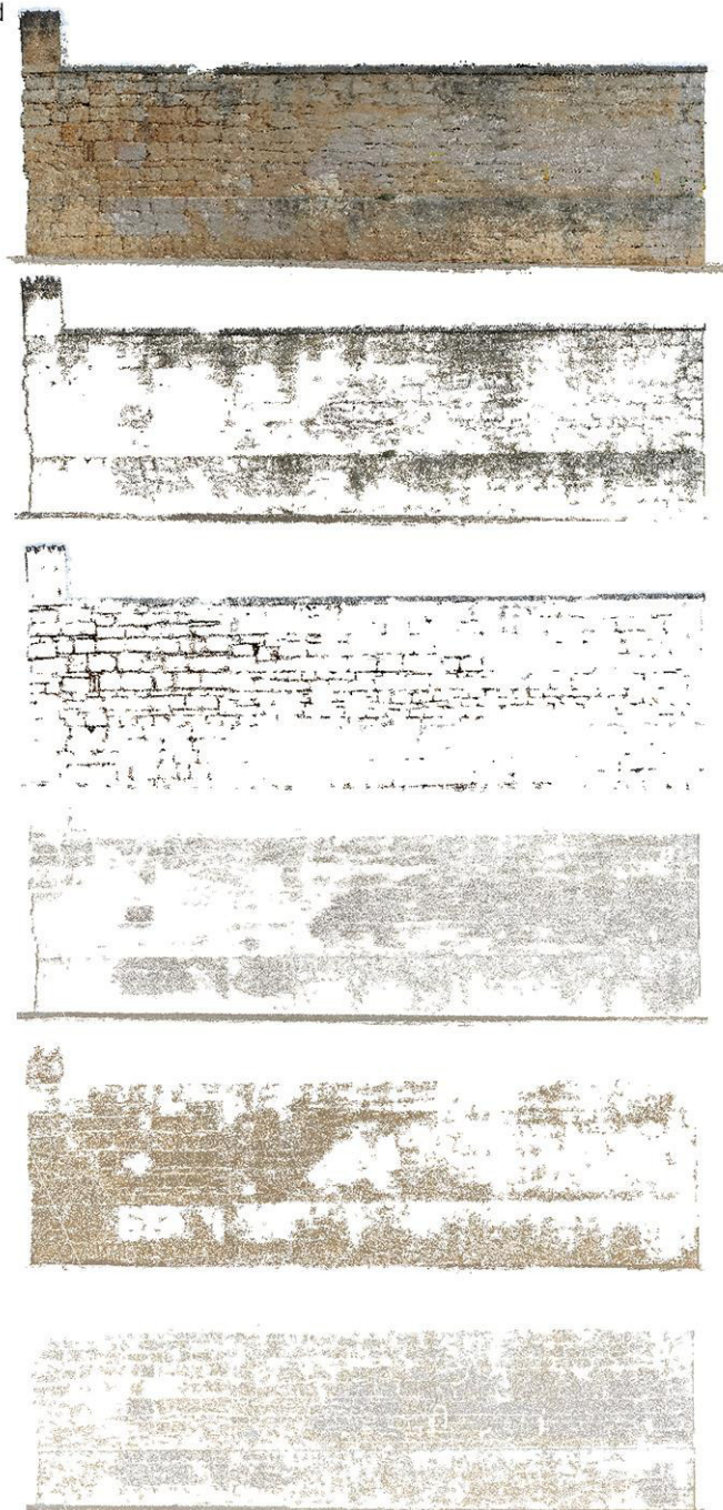
Fig. 56 Clusters in HSV (Case 3-façade Sud): 1) biological colonization (41%); 2) spots/deposit (11%);3) moist area (37%); 4) biological patina (52%) 5) unaltered surface (39%);
