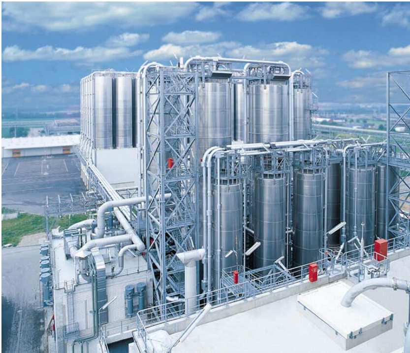
Figure 0-1 Example of plastic manufacturing plants (The photo is retrieved from the website of Coperion company)
