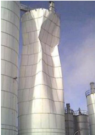
Figure 1-7 Extreme damage in grain silo caused by asymmetric flow pattern (Zaccari & Cudemo, 2016).
