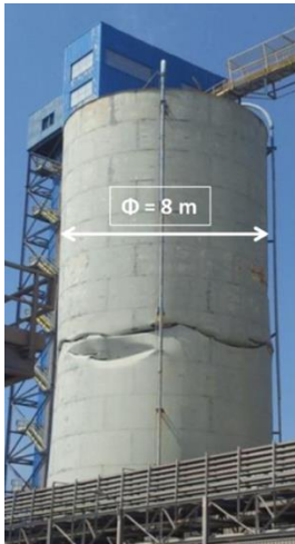
Figure 1-6 Huge shell deformation caused by buckling (Zaccari & Cudemo, 2016).
