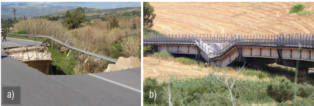
Figure 1 – Verdura (a) and Petrulla (b) Viaduct failures, Agrigento 2014
