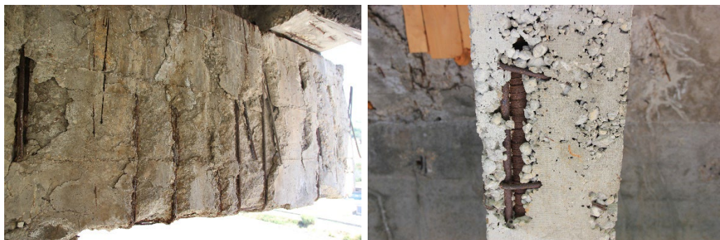
Figure 7 - Degradation of concrete structures.
