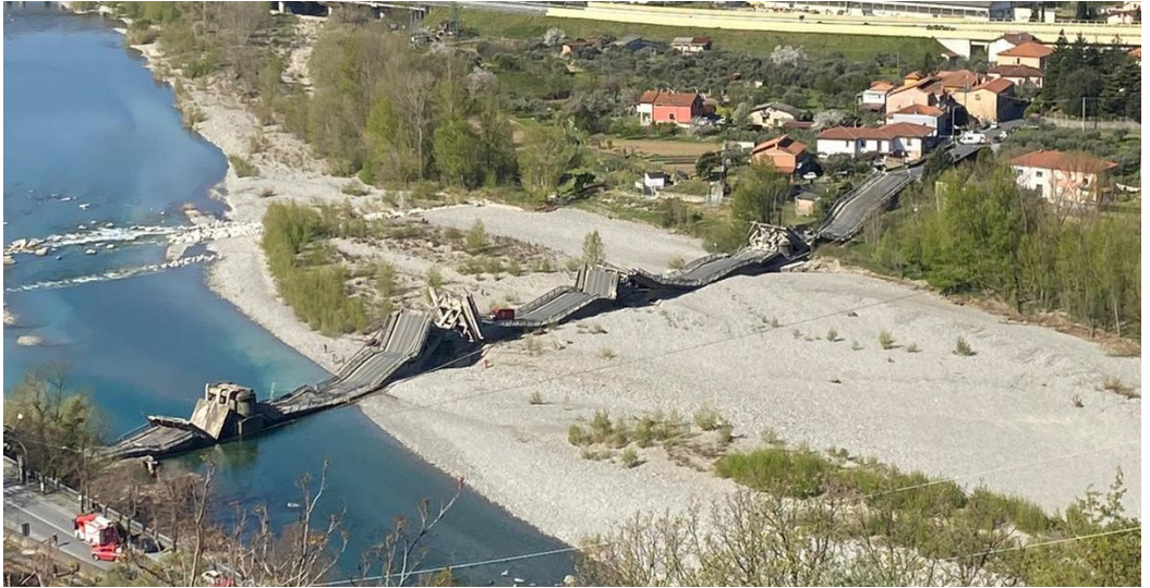
Figure 4 - Albiano Magra bridge collapse.
