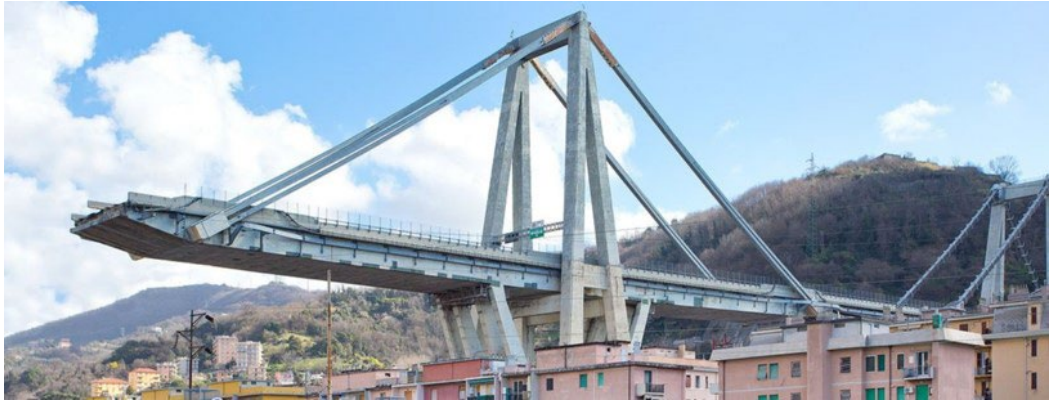
Figure 3 - Polcevera Bridge failure, Genoa 2018
