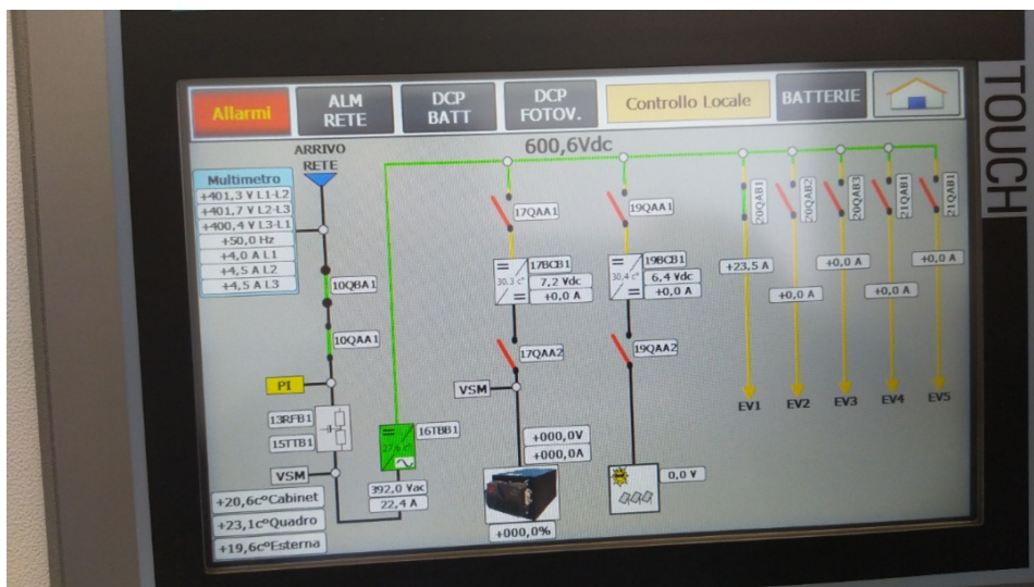
Figure 2.36: DC microgrid interface during charging test of EV1 at a V2G charging point.
