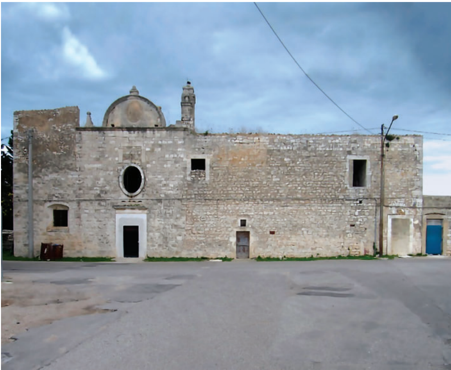
Figure 2. Conversano, the Capuchin Monastery, view of the current condition of the Western facade.
