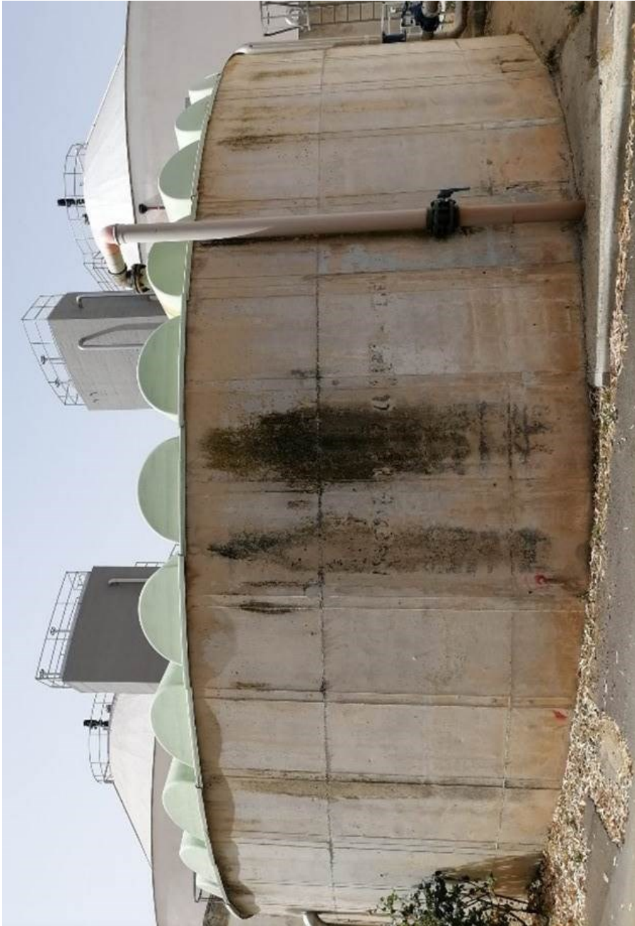
Figure S9. Static thickener and anaerobic digestors.
