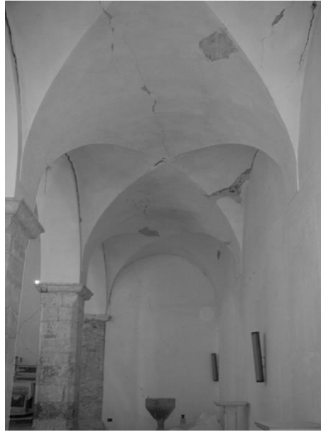
Figure 2-1. Church of San Giuliano di Puglia in Campobasso (Italy). Seismic damage (2002 Earthquake) at global scale of masonry cross vaults.
