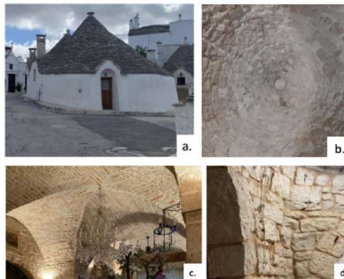
Figure 4. (a) Roughly circular plan of the modular construction unit of the trullo. (b) Interior view of the trullo pseudo-dome that forms the roof. (c) View from the inside of the juxtaposition of several modules and the detail of the junction area. (d) The thickness of dry-stone masonry on the perimeter of the trullo (photos a, c, and d by Alfonso A. Mascitelli; photo b by Giada Costa).
