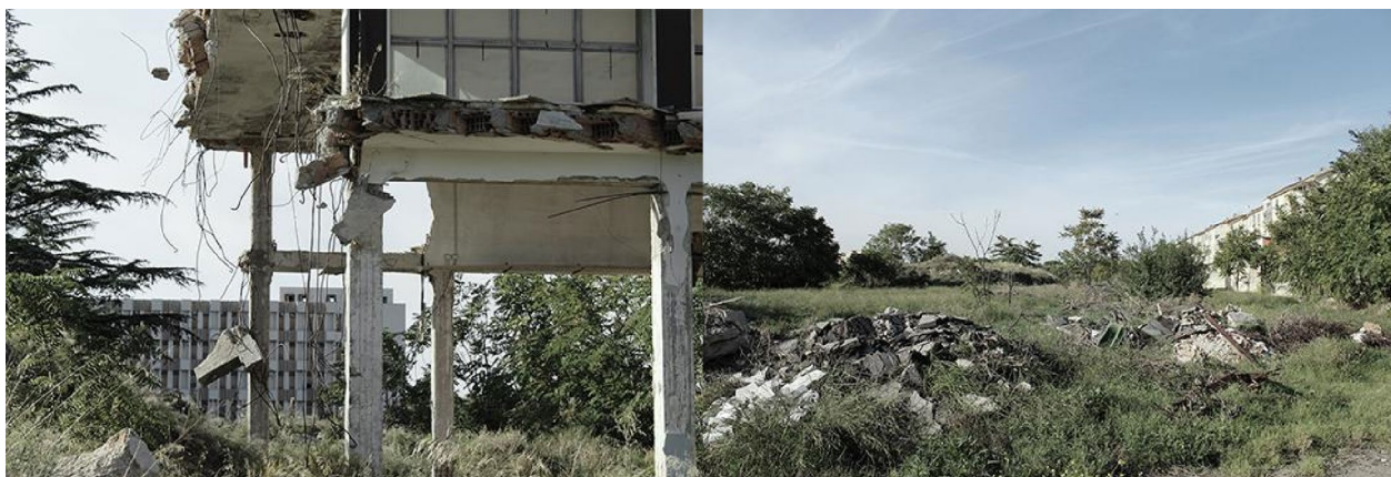
Fig. 7 Foggia, Via Lucera. Remains of collapsing buildings and waste present within the urban area of the Accordo di Programma. Source: Photo of the Authors
