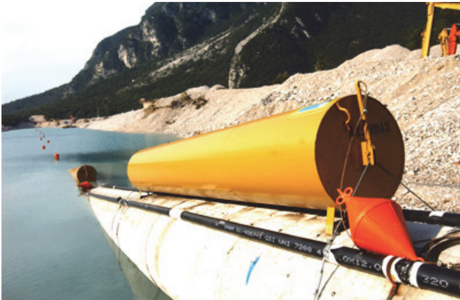
Fig. 2. Launch of a submerged methan pipe. The buoys along the launched length are in full view.
