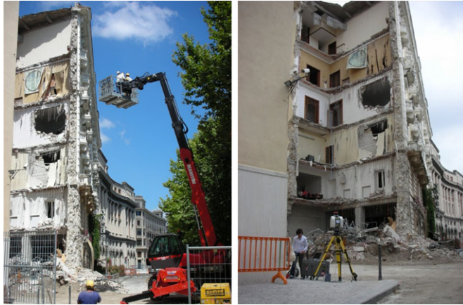
FIG. 3—Photogrammetric and laser survey with telescopic handler and station on the ground.
