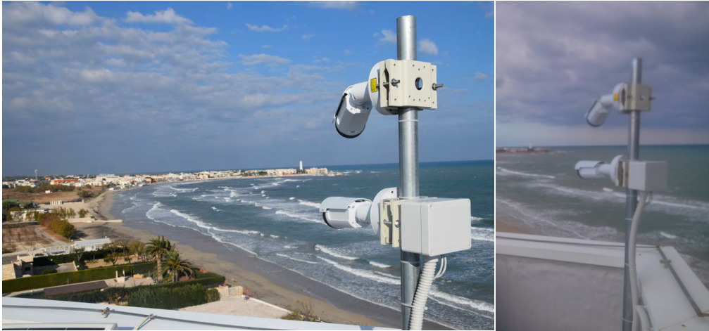
Figure 3.3 Right: Cameras location in Torre Canne (TC) and the coastal stretch framed; Left: Cameras installation.
