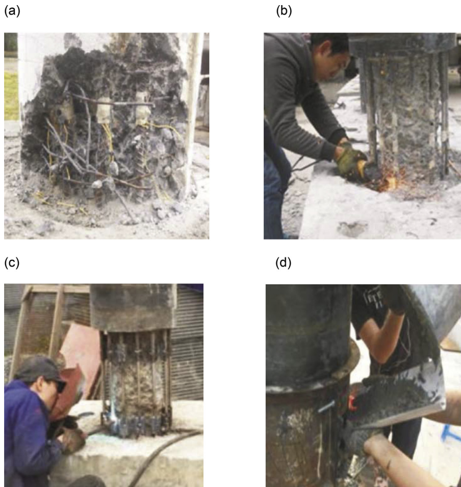
Fig. 6 – Some steps of the reinforced concrete jacketing intervention. (a) Damaged concrete removal. (b) Damaged rebar parts cut. (c) Damaged rebar parts substitution. (d) Damaged concrete cover restoration.
