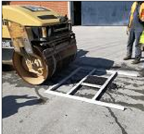
Figure 4-14 The compactor is approaching the slab which is confined in a steel frame.
