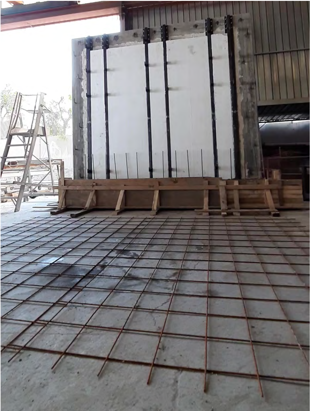
Figure E.22: Installation of the reinforcement net of the internal concrete layer of the system
