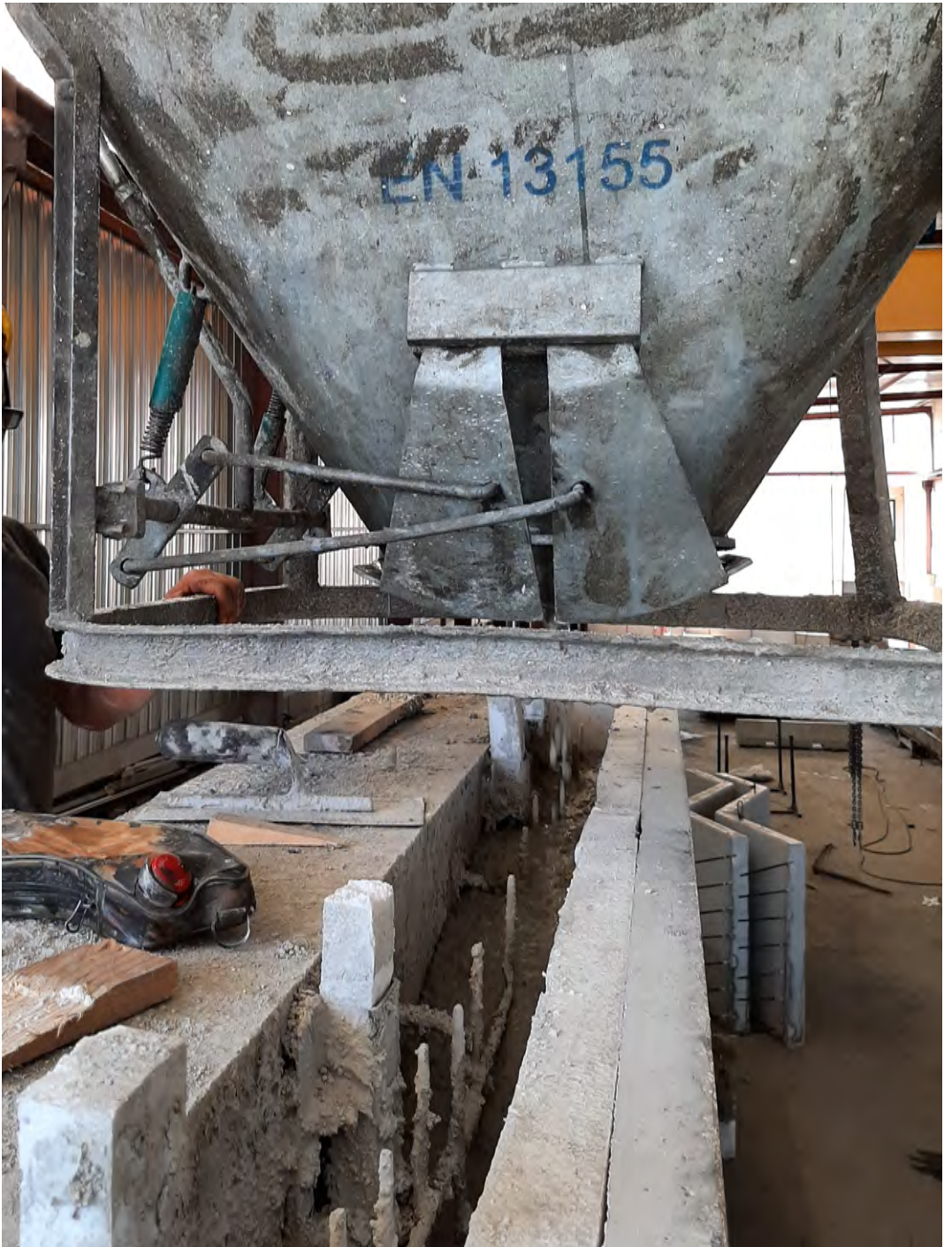
Figure E.46: Lightweight structural concrete casting in the cavity between the wall and the modules
