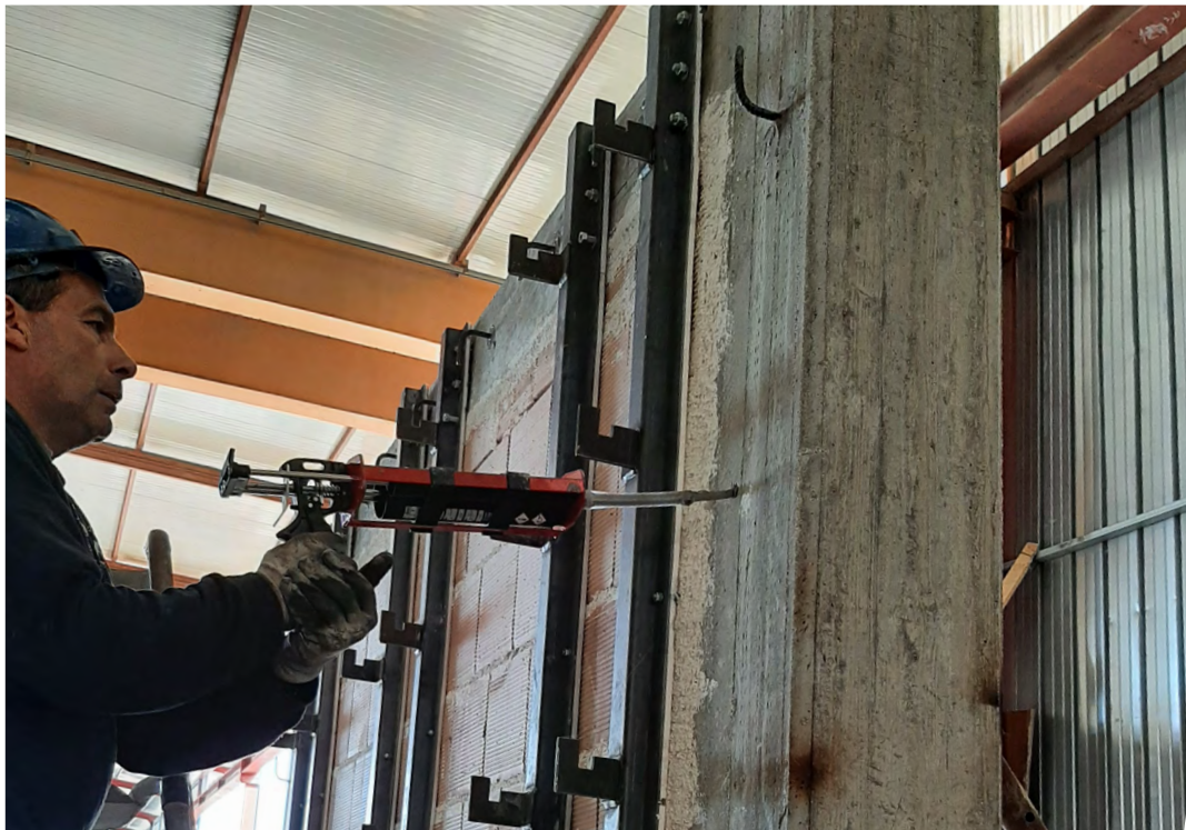
Figure E.4-5-6: Chemical injection for the fixing of the anchoris and the hooked post-installed rebars
