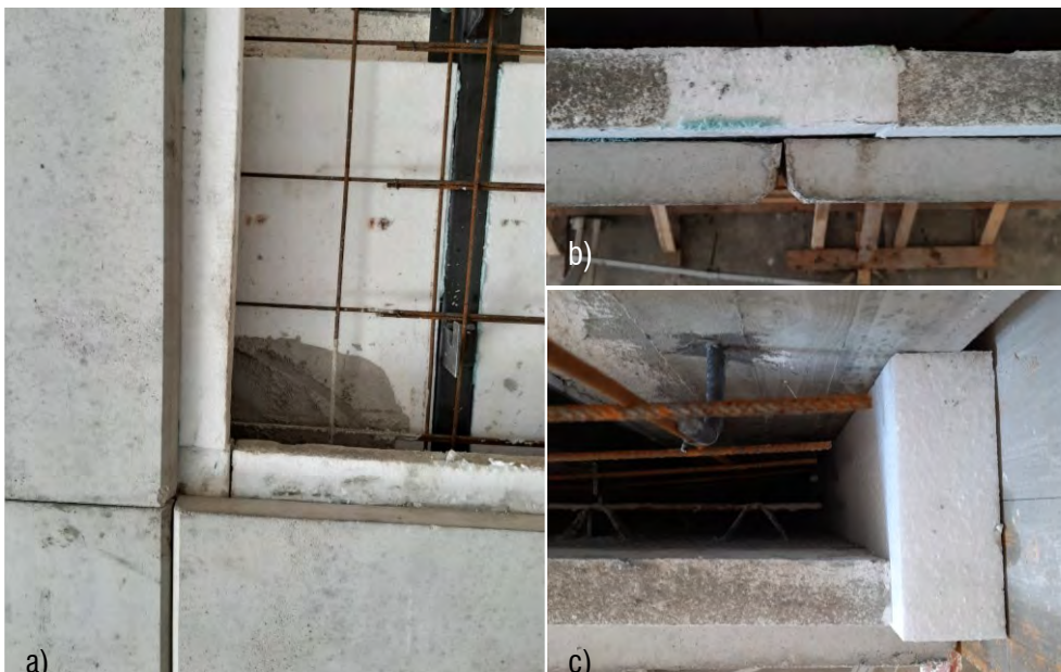
Fig. 6.3-18 – Panel layer matching: a) front view; b) two modules joint (top view); c) lateral closing of the system (top view). Source: Author
