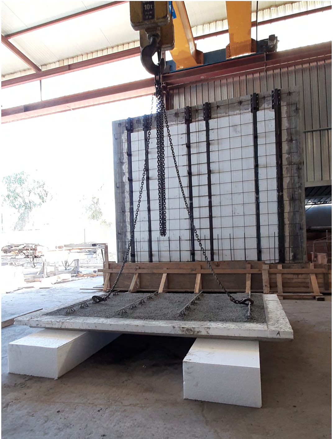
Figure E.27: Preparation for the coupling of the first PC module A to the armed wall using the bridge crane
