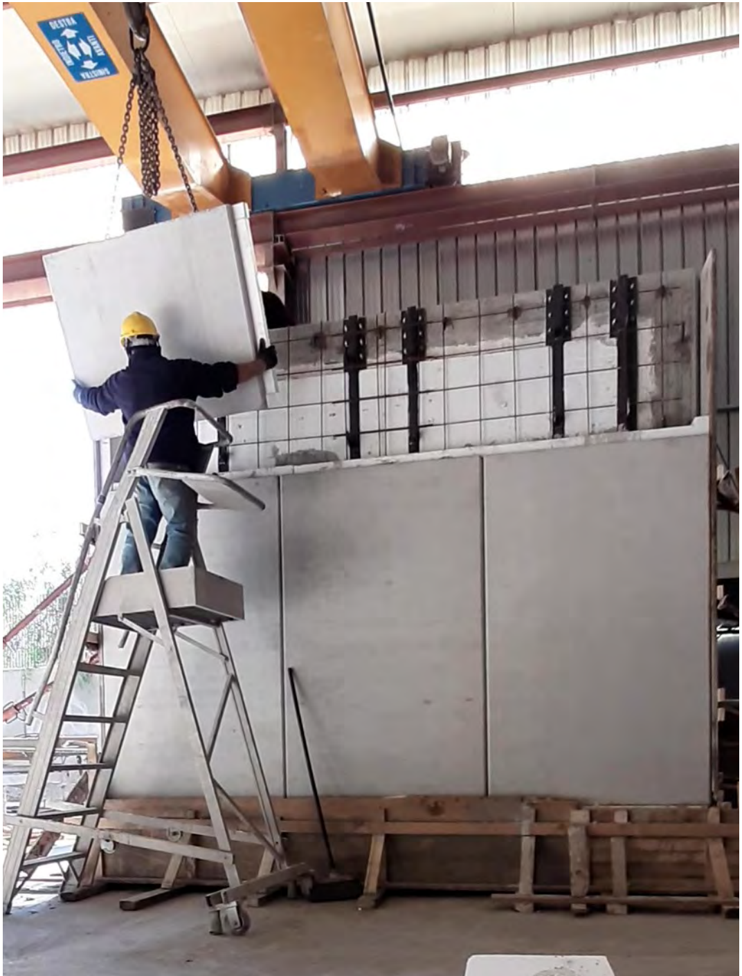
Figure E.41: Installation of the second row of PC modules (type B)
