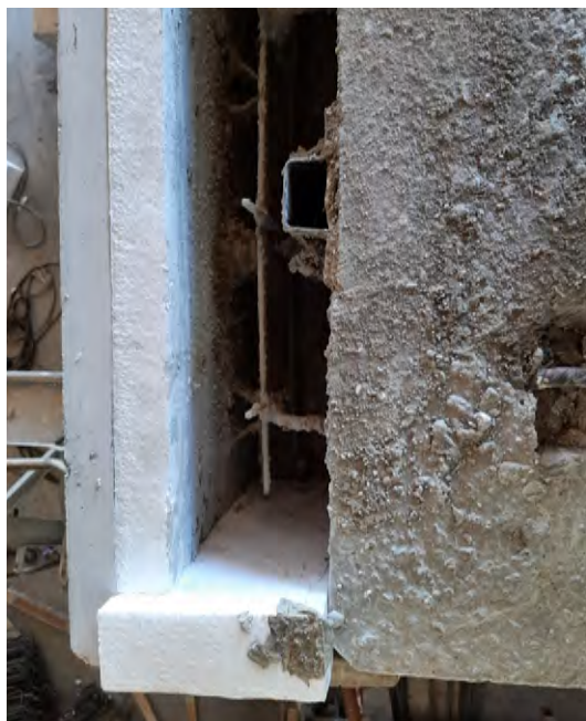
Figure E.45: Detail of the empty mullion and lateral closing of the system (top view)
