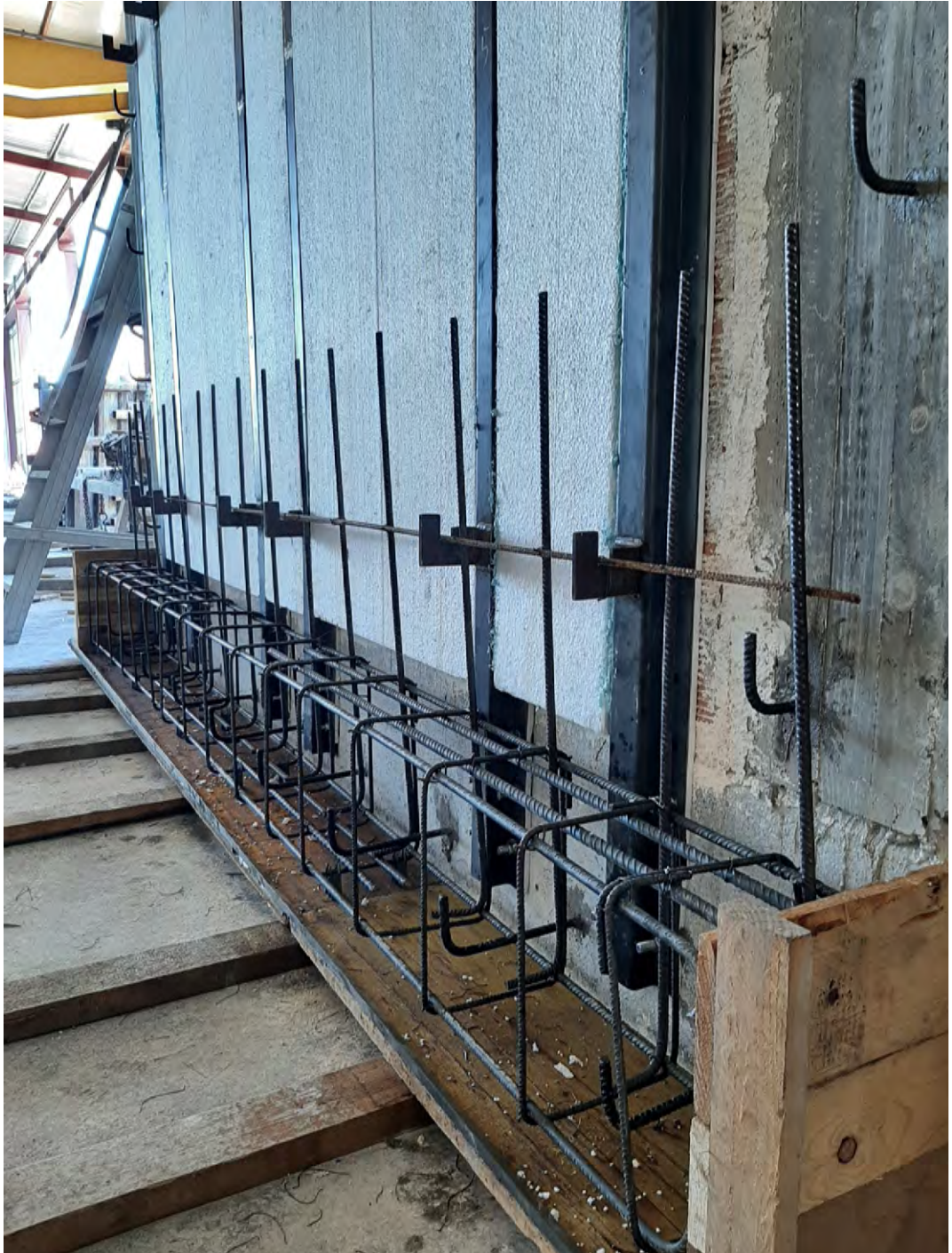
Figure E.19: Insertion of the connecting bars between the foundation and the next reinforcement mesh
