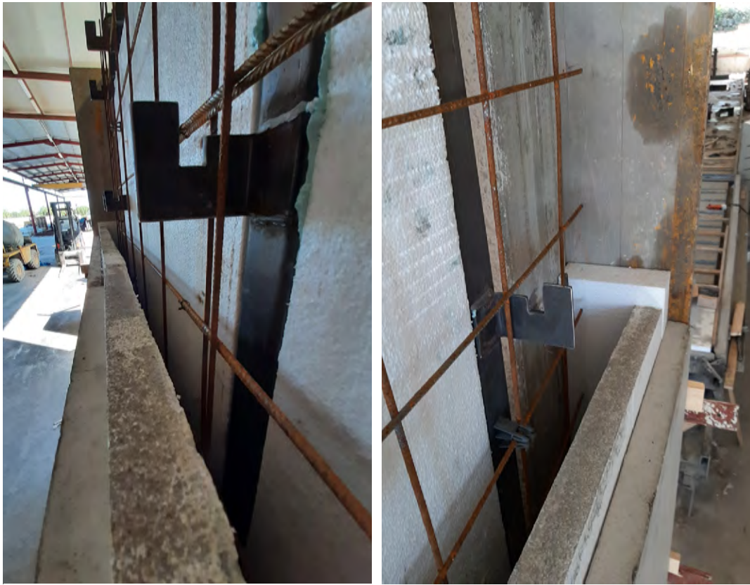
Figure E.35-36: Resulting space between the wall and the PC modules for the next concrete casting
