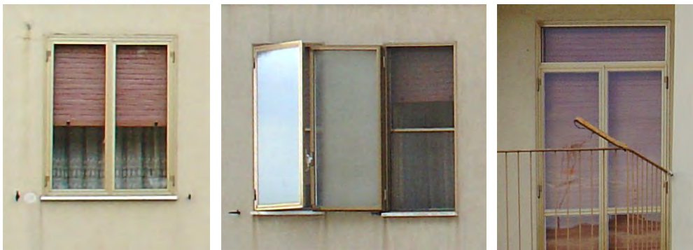
Fig. 5-2 – Case study: Survey of the windows. Source: Author
