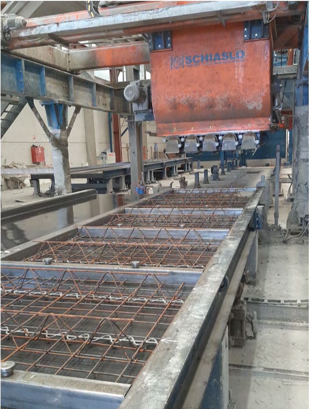
Figure B.9: Formwork moving to the concrete casting station of the carousel system
