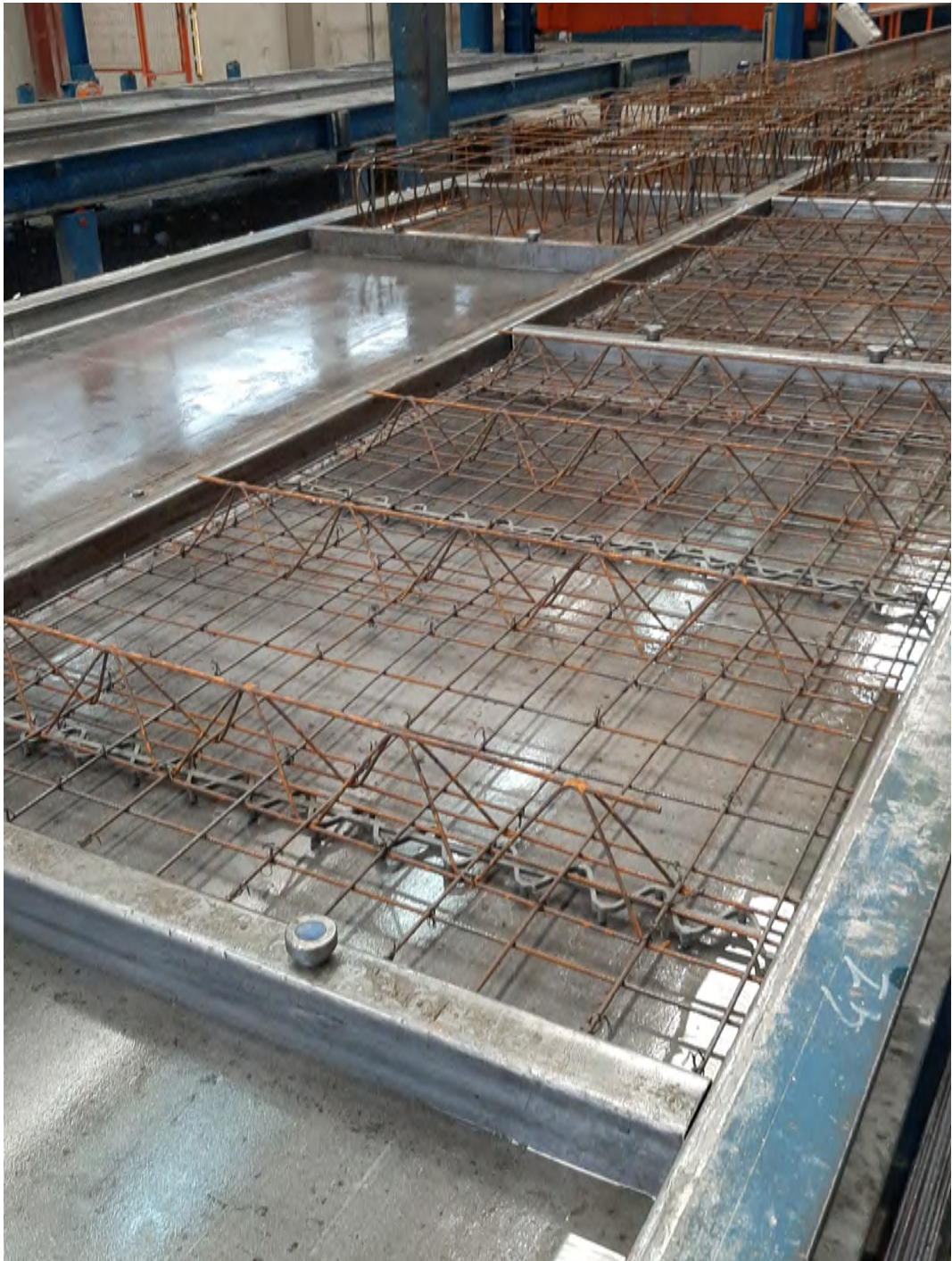
Figure B.5: The reinforcement arrangement on the formworks of the modules type A
