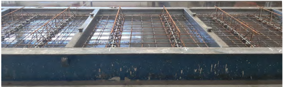
Figure B.8: The arrangement on the formworks of the modules type B: perspective view
