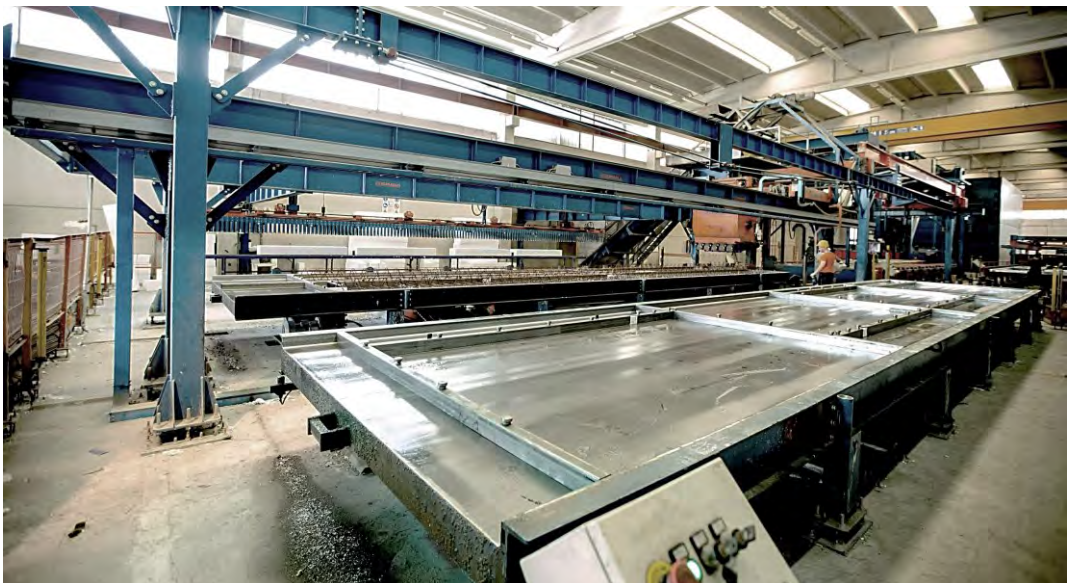
Fig. 3.4-3 - The prefabrication plant: the automated carousel system. Source: Ferramati International s.r.l.
