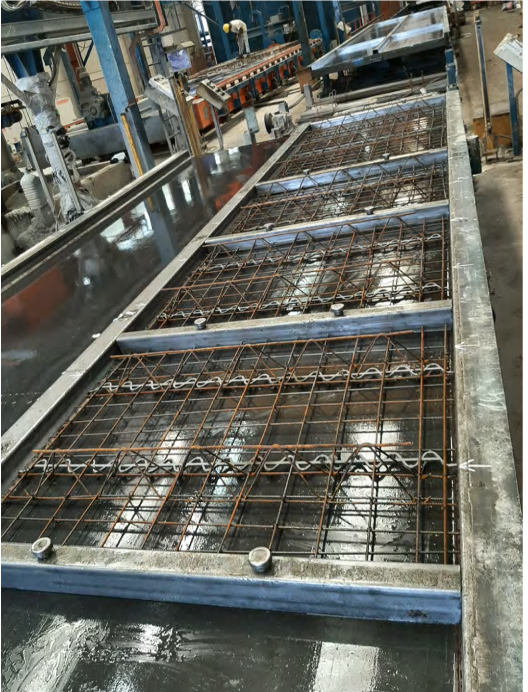
Figure B.6: The reinforcement arrangement on the formworks of the series of modules type B
