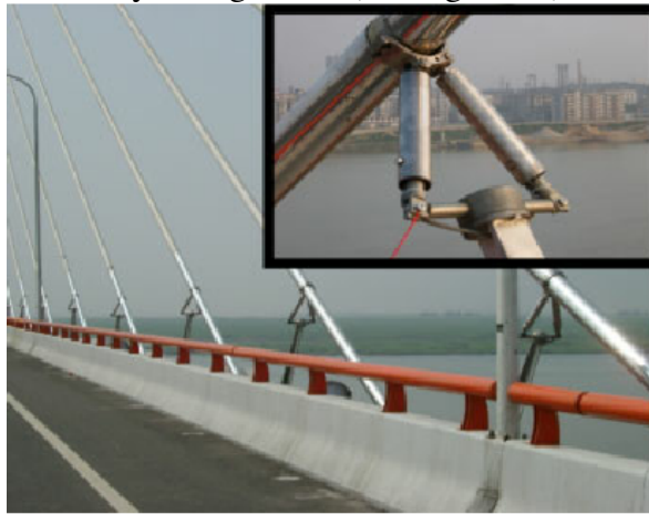
Figure 43. The MR dampers connecting the cables and the deck of the bridge on Dongting Lake, China. [ https://goo.gl/VUhKDO ; access on 07/01/2021] [139].
