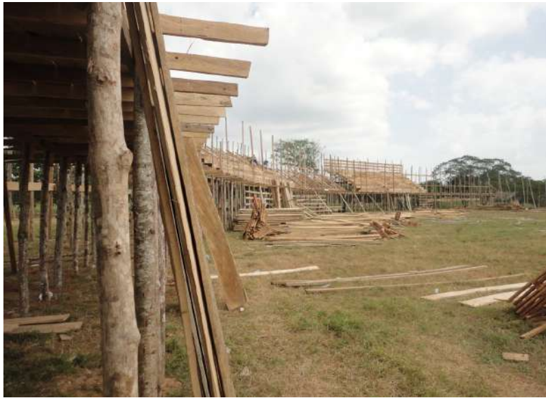
Figure 11. Image of the assembling of a Corraleja , where the main constructive elements are evident. Source: Merwan Chaverra, 2017 [14].
