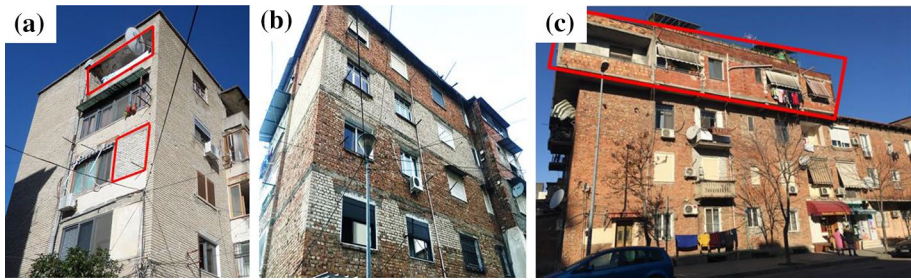
Fig. 19 Unauthorised interventions on unreinforced masonry (URM) buildings in Durrës. a Irregularities in the opening layout due the closure of part of the balcony; b use of different construction materials and c presence of an additional floor
