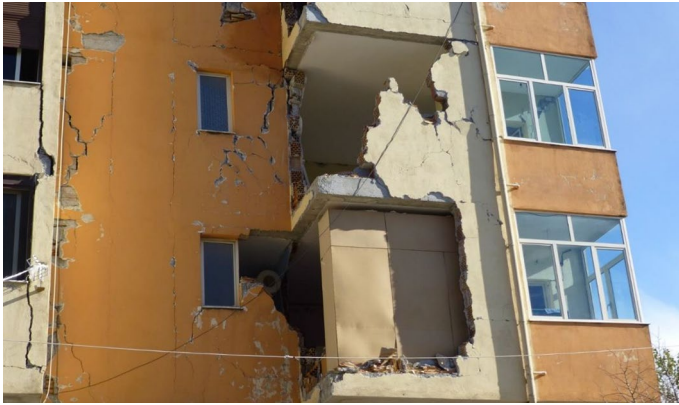
Fig. 13 Typical 2000s multi-storey reinforced concrete (RC) building compliant with KTP-N.2-89. Damage layout in the eastern façade of the building
