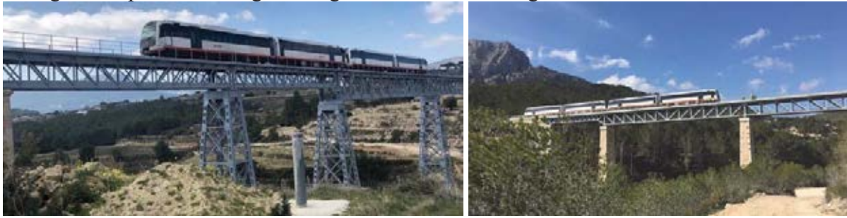
Figure 1. Two examples of old steel bridges in the Valencian railroad network: “Quisi” (left) and “Ferrandet” (right) bridges.
