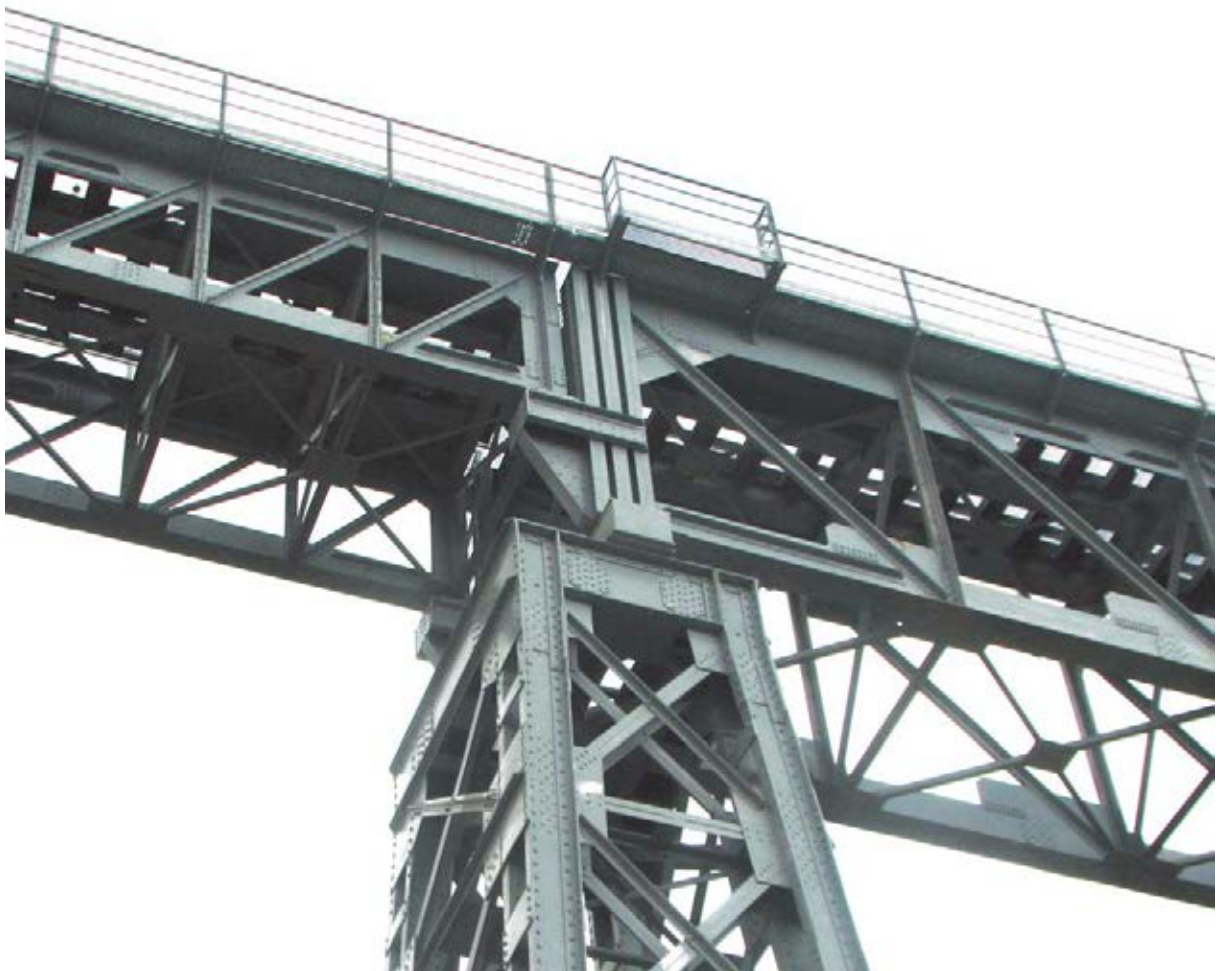
Figure 6: Connection between the isostatic span 2 (left), the hyperstatic span 3 (right) and the steel tower.
