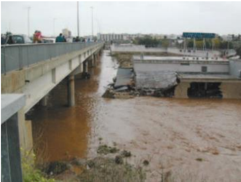
Figure 2.17 Collapse of the building of a company of the S. Rita flyway after 2005 flooding event
