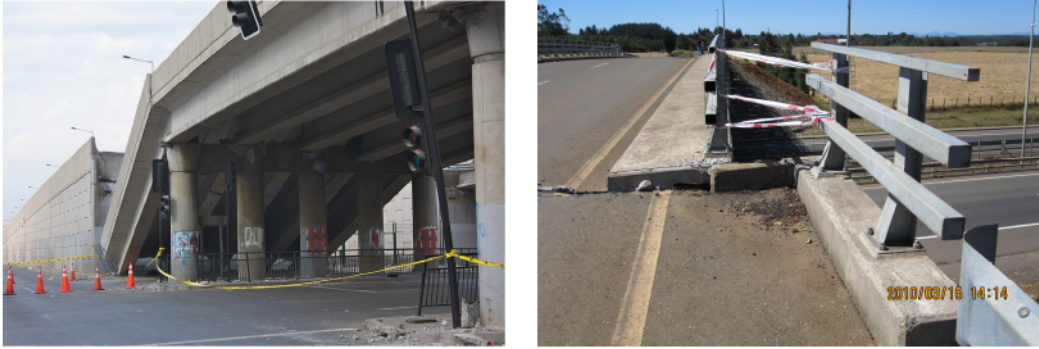
Figure 1.4: Failures of roadway bridges during the Chilean earthquakes 2010 https://www.flickr.com/photos/38631801@N07/4404042277 and http://learningfromearthquakes.org/2010-02-27-chile/images/2010_02_27_chile/
