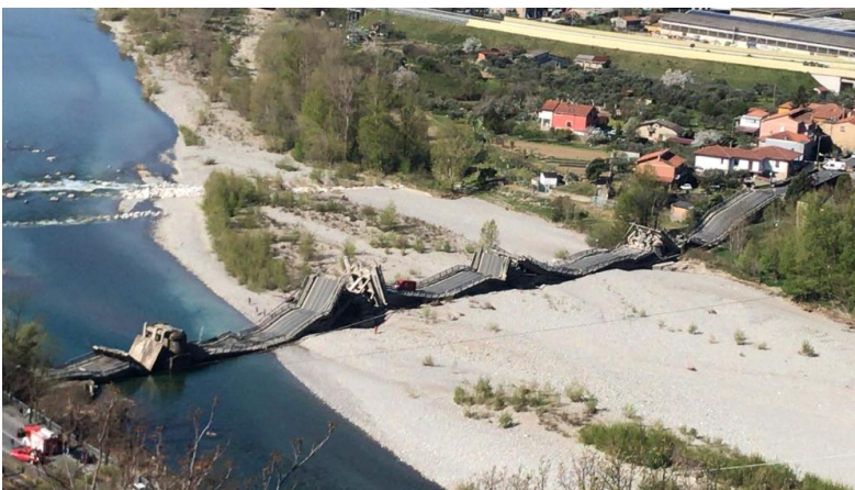
Figure 1.2: Collapse of a bridge in Albiano Magra (Massa-Carrara, Italy), 8th April 2020
