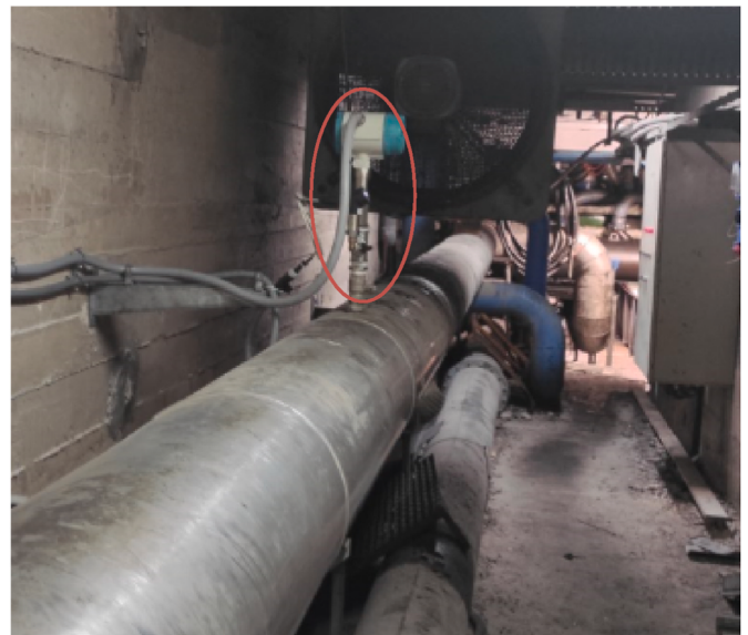
Fig. 4. Installation of the thermal flow meter on a compressed air line of the plant.
